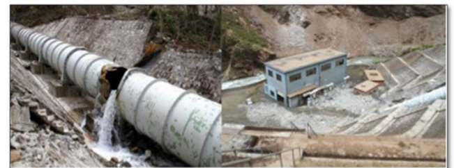
Fig. 3: Bhoté Koshi hydropower plant in Sindhupalchok, Nepal
