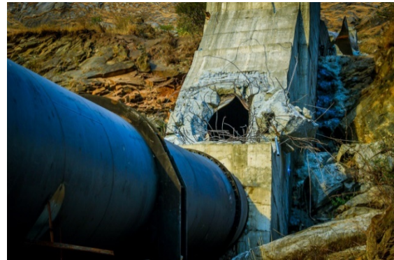
Fig. 2: Penstock burst at Sorang Hydropower Project in Himachal Pradesh, India
