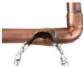
Fig. 6: Water hammer damage to domestic pipe
