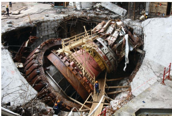
Fig. 1: Wrecked turbine at Sayano-Shushenskaya hydropower plant in Siberia
